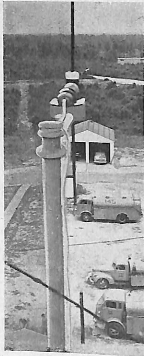
ANTENNA INSTALLATION on control tower roof, showing proximity of this antenna to vehicles having unshielded ignition systems.
