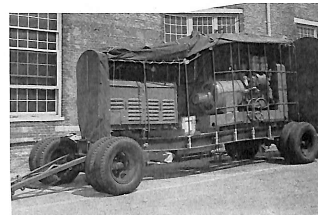
Mobile communication power trailer, U. S. N. 193440. Showing PE-95G and 75 kw Diesel-driven generator.
