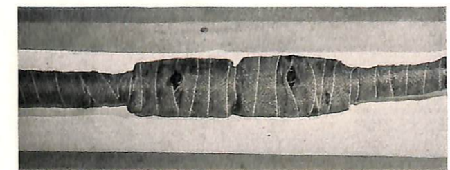
FIGURE 12—Completed splice wrapped in jute tape and ready for the application of the Okonite compound.
