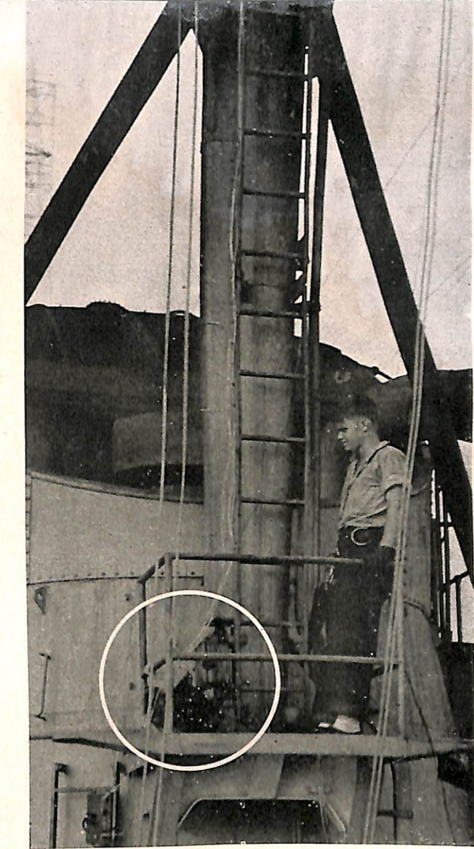
Closeup of the Wisconsin's insulated-duct installation. Note the blower motor at the lower end of the duct.
