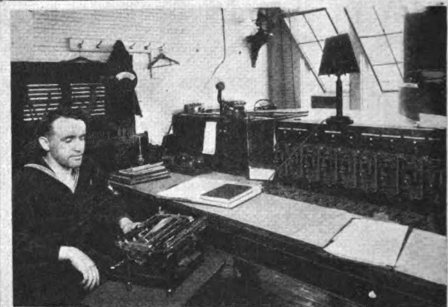
In the left background of the above photo may be seen the switchboard connecting with various points along the Atlantic coast. On the right hand side of the picture are the relays and keys used in connection with these lines.
