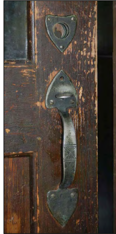
Figure 53a. Extant Suffolk-style latch and escutcheon on interior door to NE Hallway vestibule. Note the similarities to the hardware in the catalog illustration.
