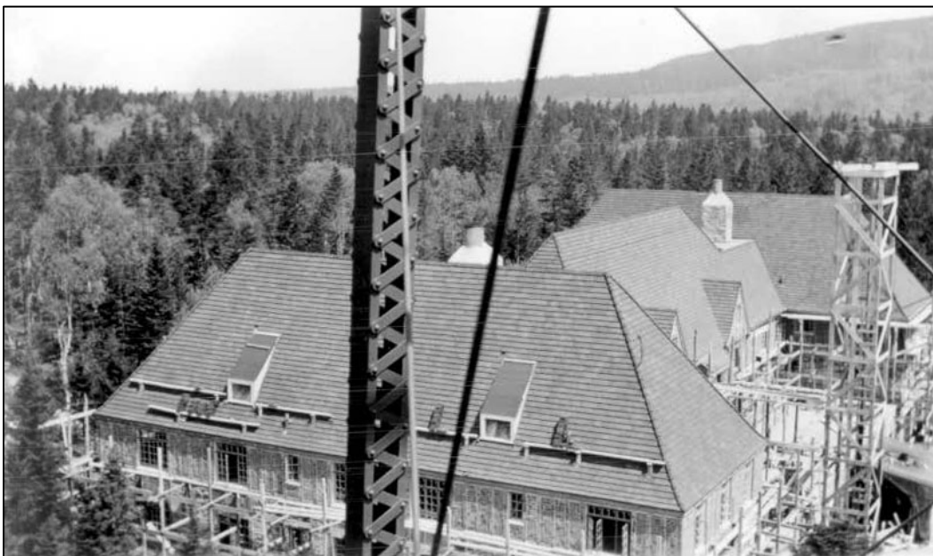
Figure 27. Apartment Building roofs, looking north with Southwest Pavilion in foreground, photograph taken from south radio tower, June 2, 1934.
