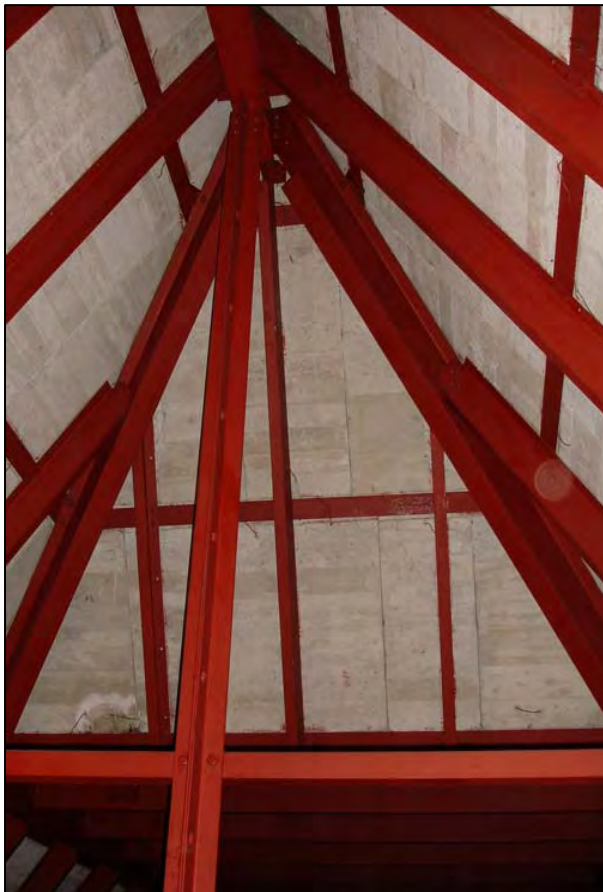
Figure 70. Apartment Building typical steel framing of hipped roof and "nailcrete" sheathing panels, 2008.
