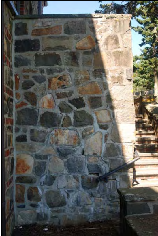
Figure 50. Apartment Building, Northeast Pavilion, SE wall of NE entrance stoop to D108, 2008.
