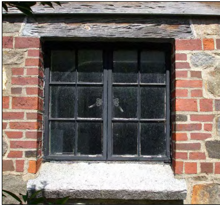
Figure 35. Power House, SE elevation, window opening with brick jamb, granite sill, pecky cypress lintel, and steel casement sashes, 2008.
