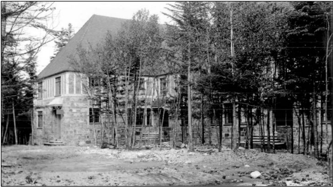
Figure 17. Apartment Building, NW elevation courtyard before grading and topsoil was deposited, November 1934.
