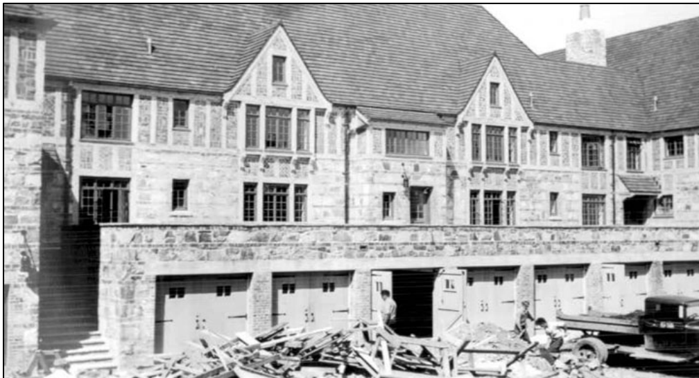
Figure 26. Apartment Building, SE elevation depicting window openings with original multi-light steel sashes, September 1934.
