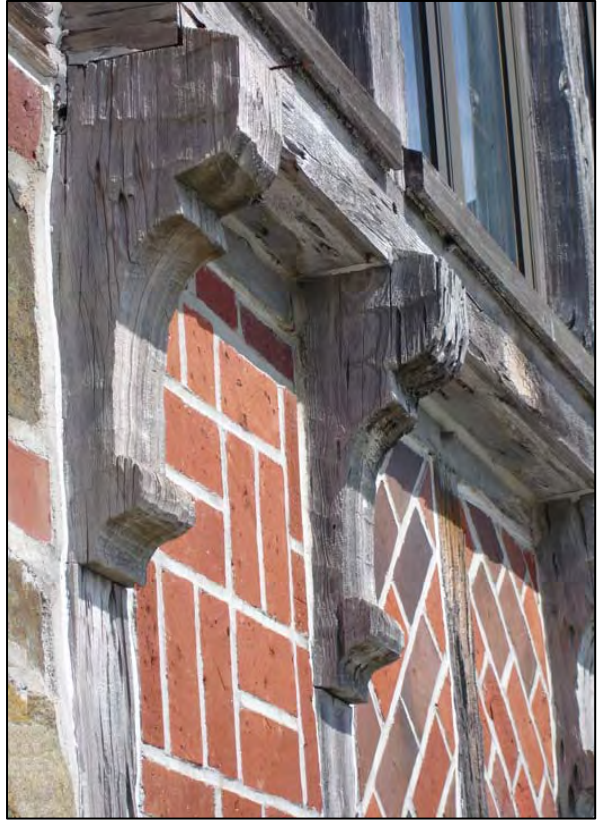
Figure 48. Apartment Building, SE elevation, well preserved cross-gable brackets supporting second-story window opening bay, 2008.
