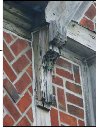
Figure 47a. Apartment Building, SE elevation, deteriorated cross-gable bracket, 2008.
