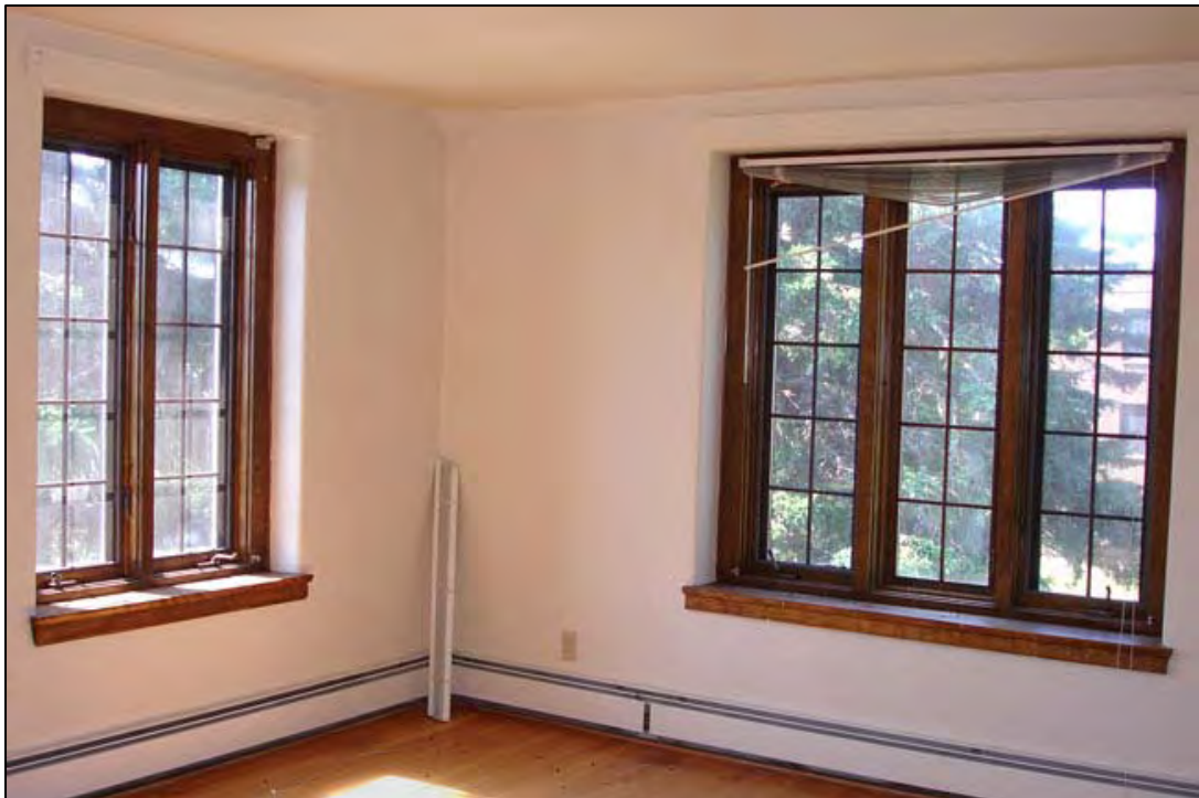
Figure 64. Apartment Building typical interior of window openings with two sashes (W227) and three sashes (W226), 2008.
