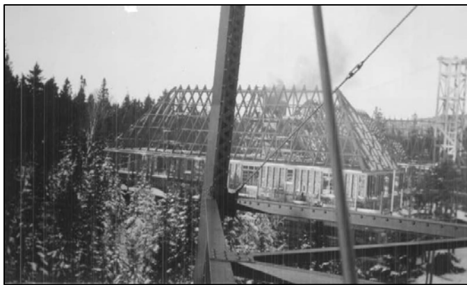
Figure 11. View of the SW elevation and roof framing from SW radio tower, December 9, 1933.
